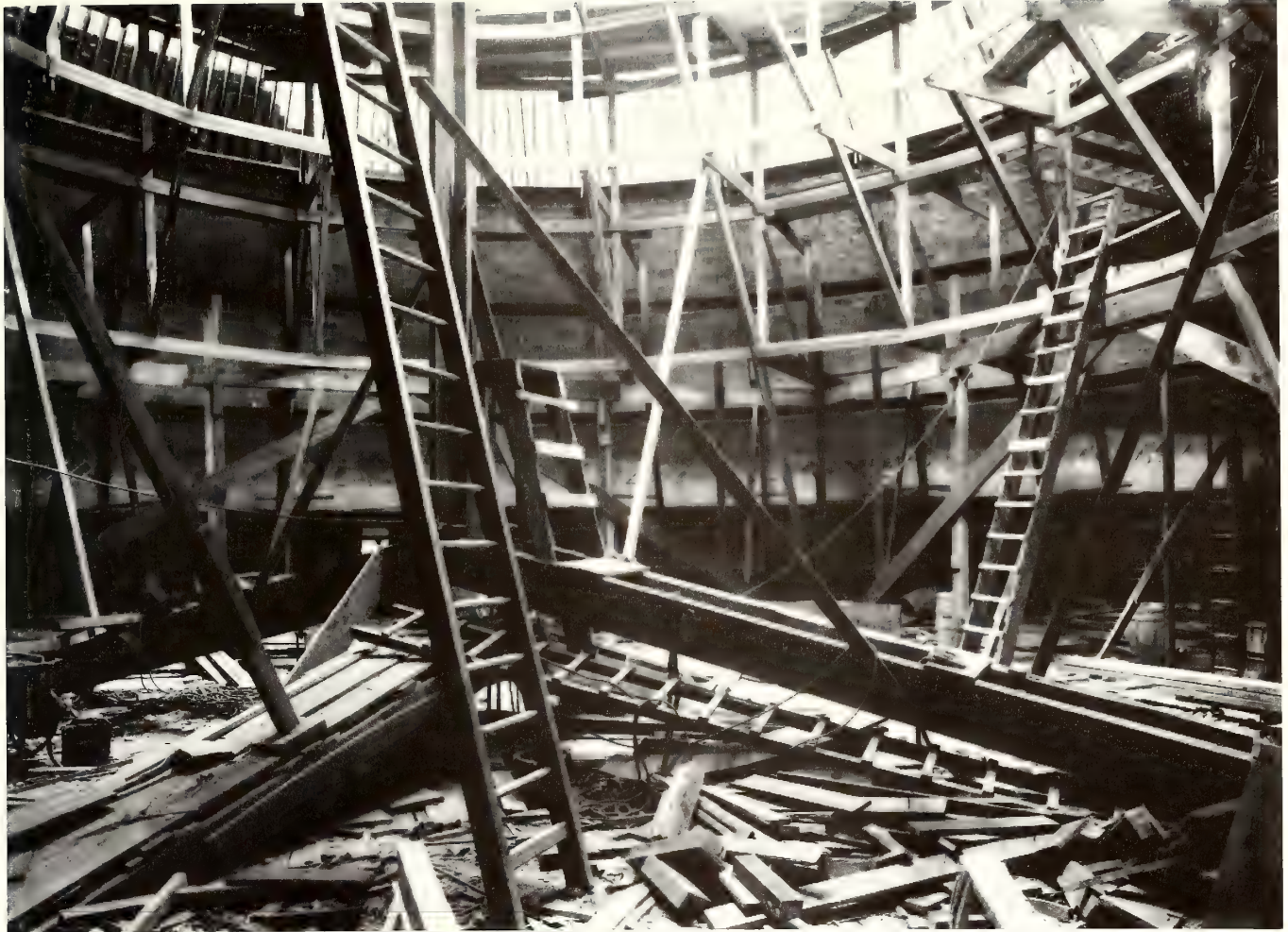
Building the dome, probably 1910. Workmen built this wooden floor and then erected scaffolding to construct the inner dome. The inner and outer domes rest on brick piers
